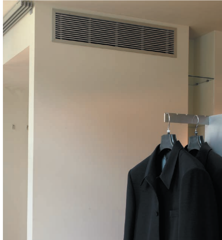
Concealed ceiling unit
